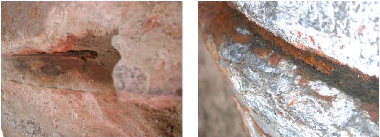
Figure 5: Failed PCCP Joint in Luck Lake, SK
