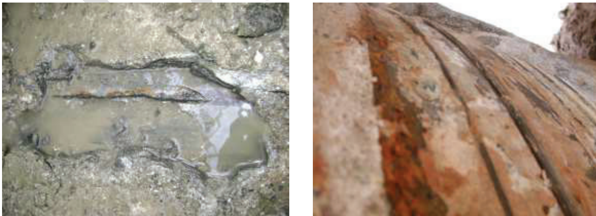
Figure 6: Luck Lake, SK - Progression of Joint Deterioration to Prestressing Wires
