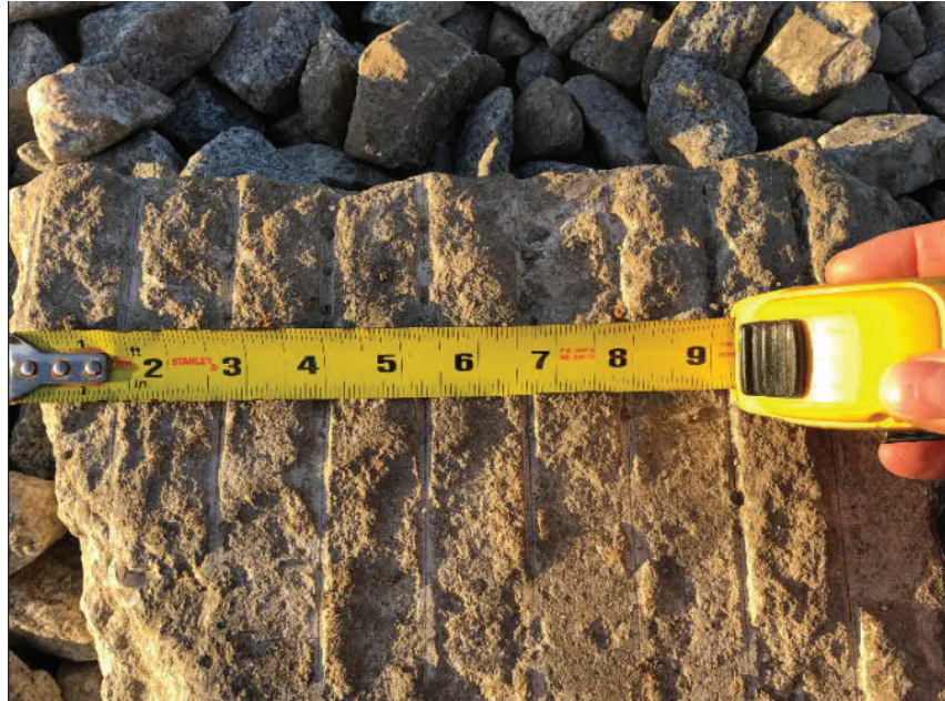
Figure 2: Underside of Mortar Coating from PCCP, Revealing Wire Diameter and Spacing.
