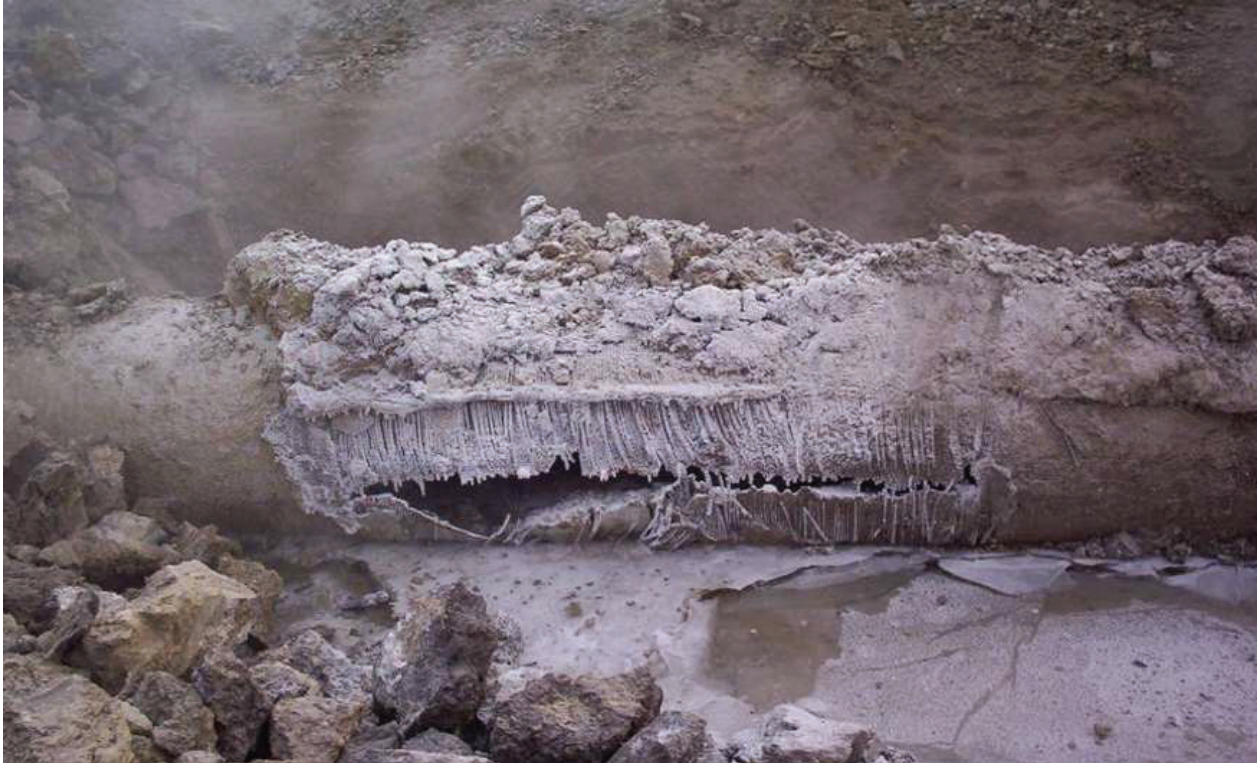
Figure 4: PCCP Barrel Failure - McKnight Blvd and Resultant Loss of Water, Calgary, AB
